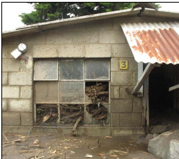
One house is half-filled with sludge and branches washed in. This window previously stood four feet off the ground.
